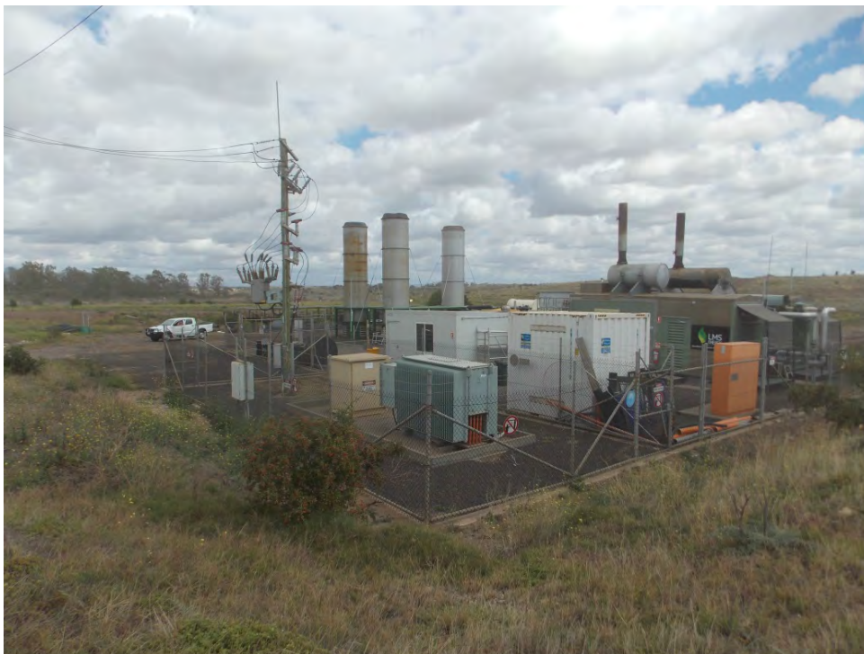
Figure 7 Biogas power generation plant
